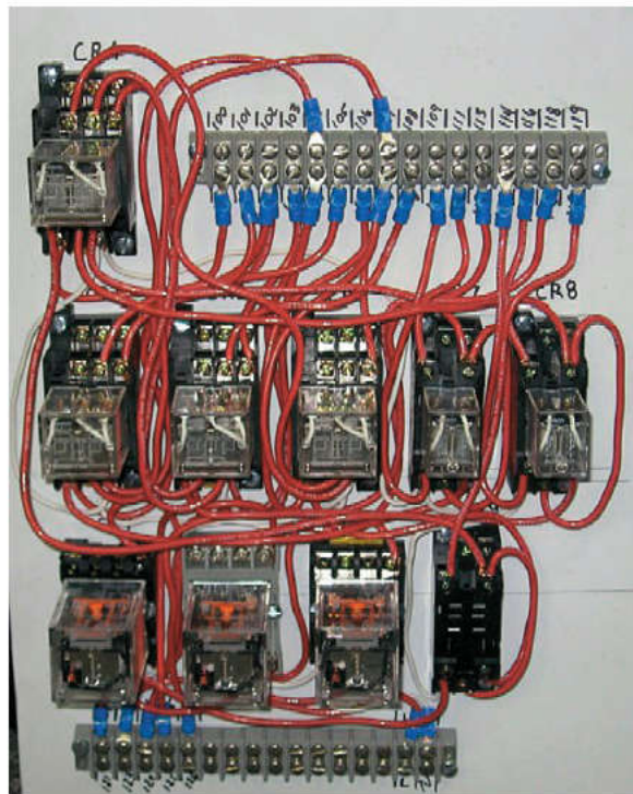
Relay control panel
