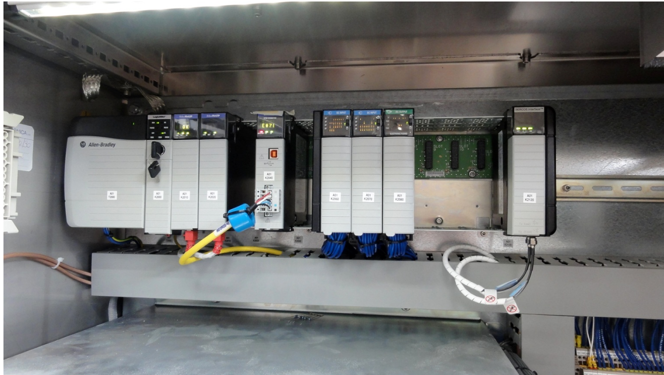
1 of the PLCs used by A3/Flex (Allen-Bradley PLCs)
