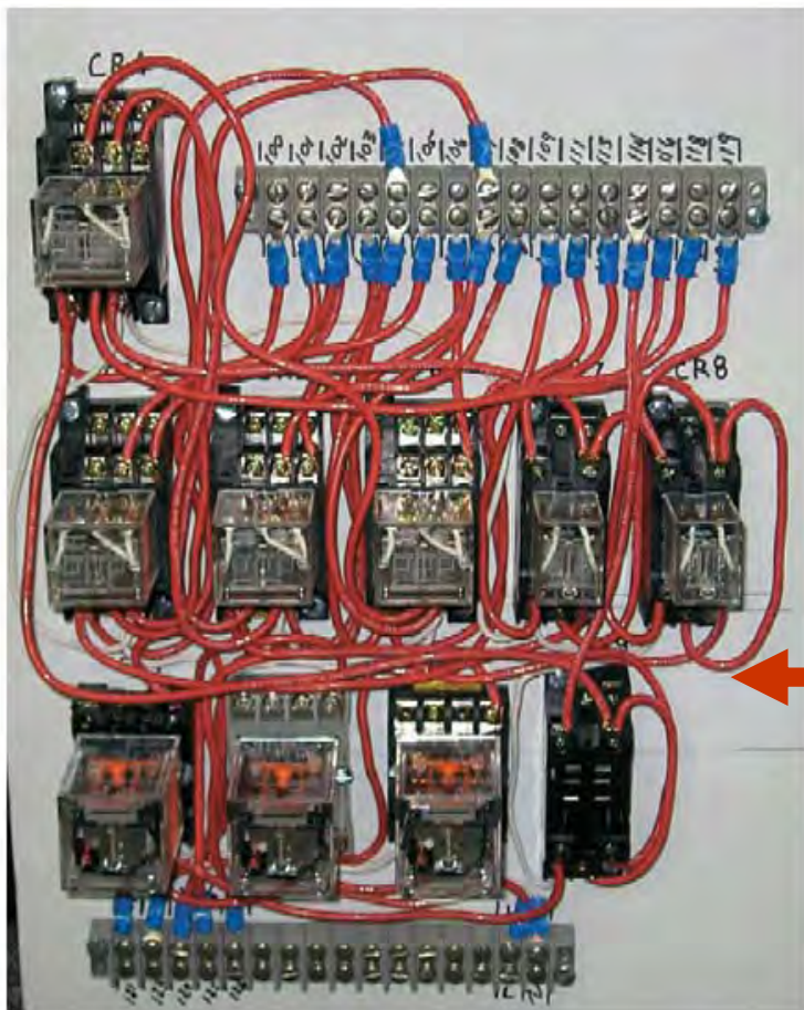
Relay control panel
