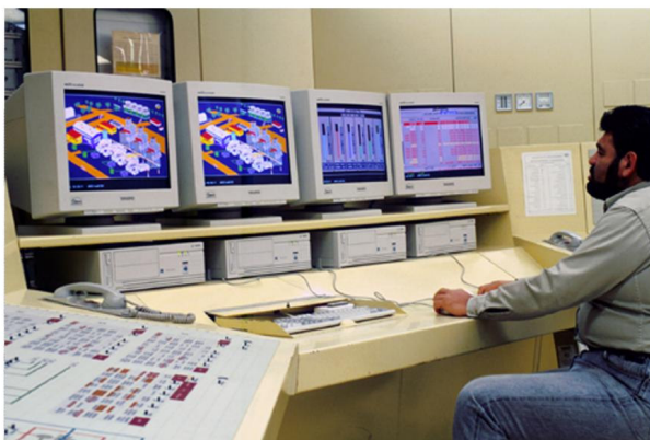
Fig2. Plant operator console
